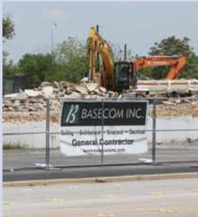
Work has begun on the removal of key concrete slabs to make way for new TRV bridges at Henderson St. and White Settlement Rd.
