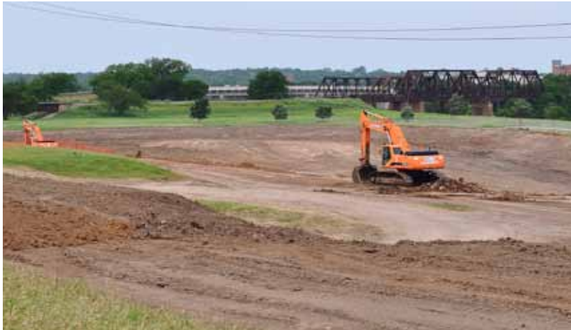
The Penna Group will move approximately 45,000 truckloads of dirt near Northside Dr. and Samuels Avenue for the US Army Corps of Engineers
